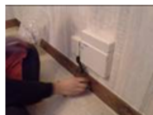
Inkoppling i switchen
